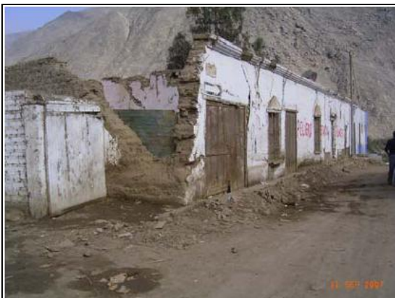
Collapse of adobe building corner, Cañete river valley, Peru, September 2007. Courtesy of EEFIT
